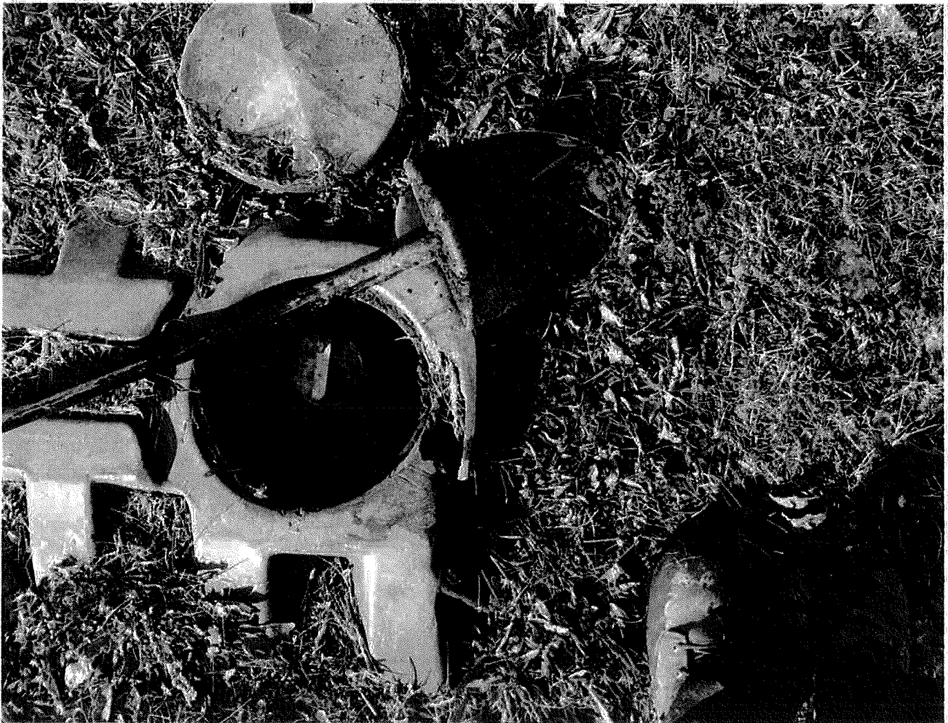
Break in 2nd septic tank
